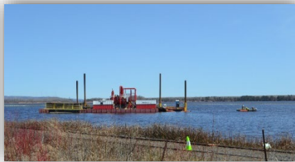
Capping in the Wire Mill offshore and Unnamed Creek offshore areas was completed in June 2022. Capping is ongoing in the SSB over the dredged surface.
