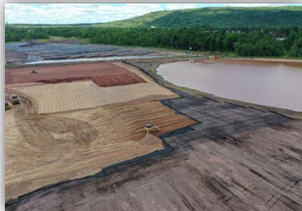
The Delta Upland Cap is being constructed adjacent to the SSB. The cap area will support recreational features designed in coordination with the City of Duluth.
