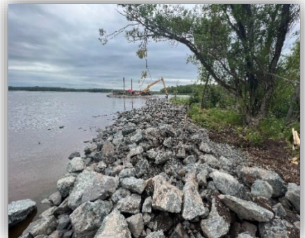
Placement of rock for shoreline protection is ongoing along select sections of shoreline within the project area.
