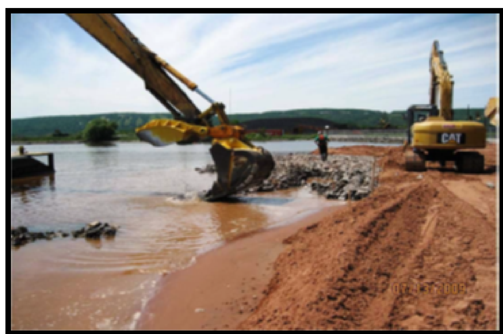
7cbWdhi U'example of cap armor placed along a shoreline.
