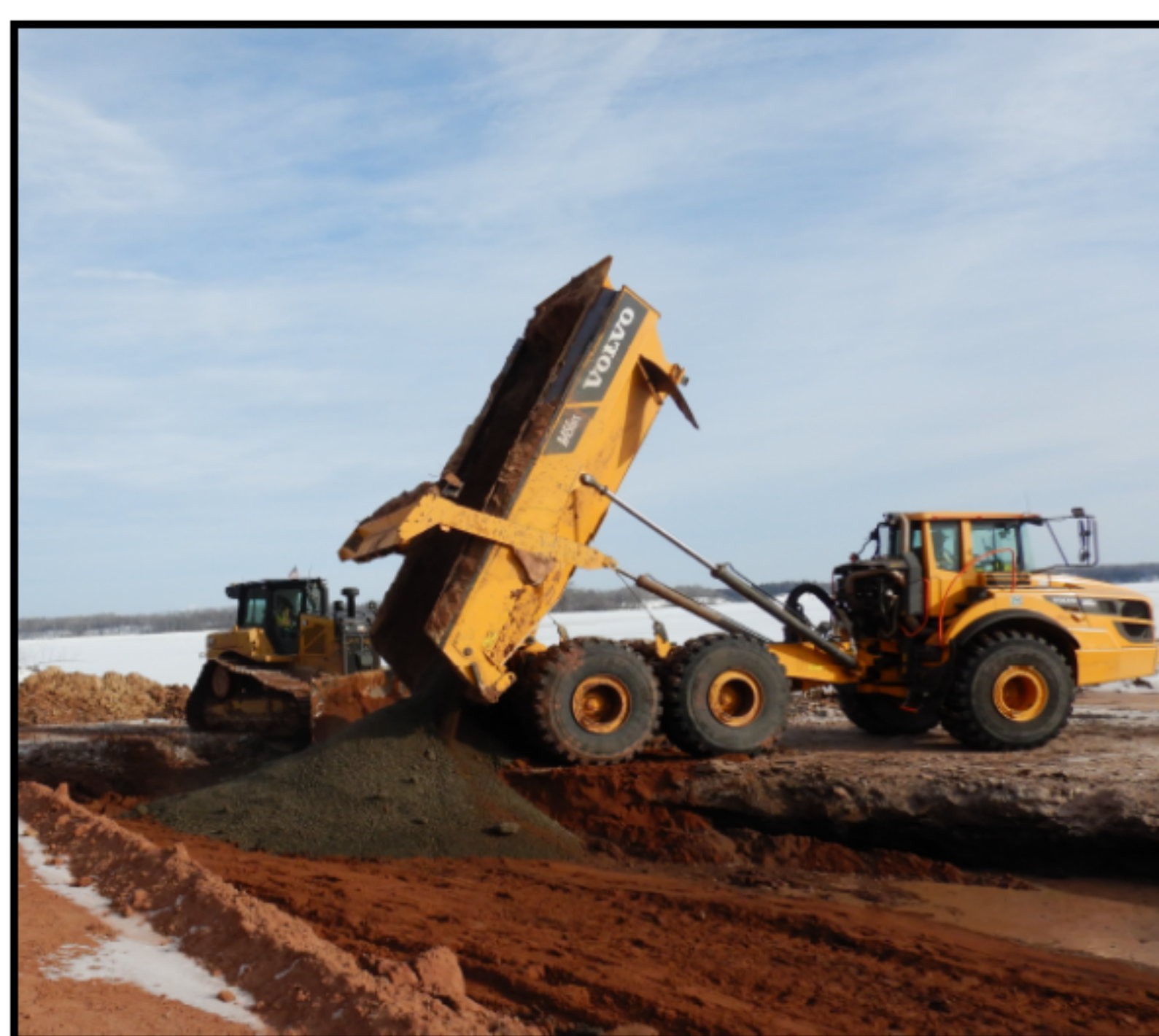
Root barrier being installed in a cap in the Shallow Sheltered Bay Spirit Lake.
