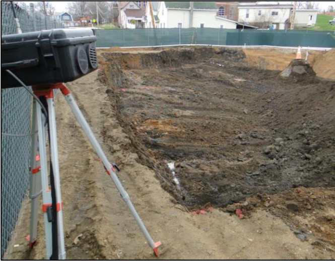
A typical perimeter air monitoring station that will be used to track airborne pollutants and dust.
