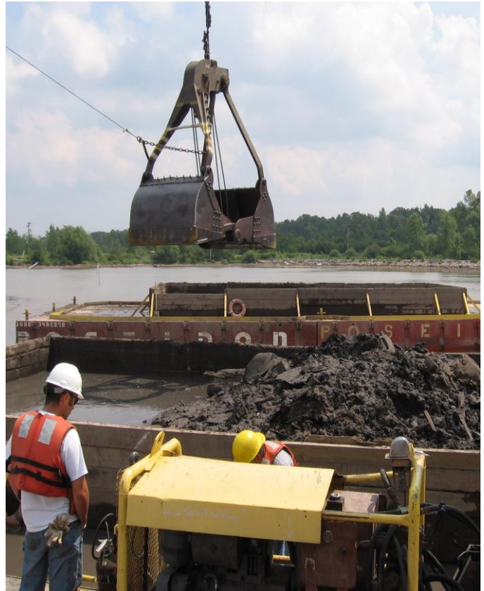
A dredge deposits sediment dug out of Tannery Bay onto a barge. Workers removed the water from the mud, treated the water and disposed of the contaminated
