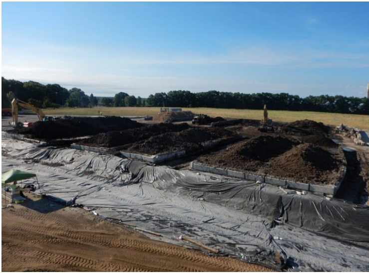
Sediment is temporarily placed at the staging area for drying (dewatering) prior to transport to a landfill for off-site disposal.
