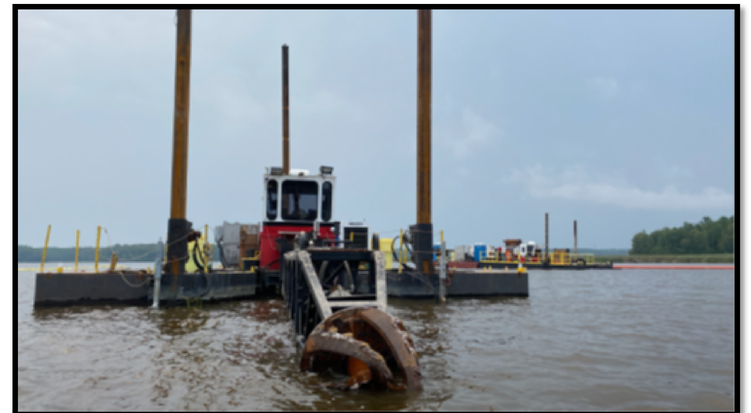
Dredging is conducted with a hydraulic cutterhead dredge in the Wire Mill Delta.
