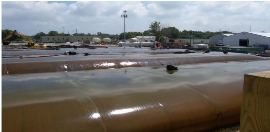
Geotubes (photo above) are pumped full of wet sediment (mud) during dredging. Geotubes trap contaminated sediment and drain excess water.
