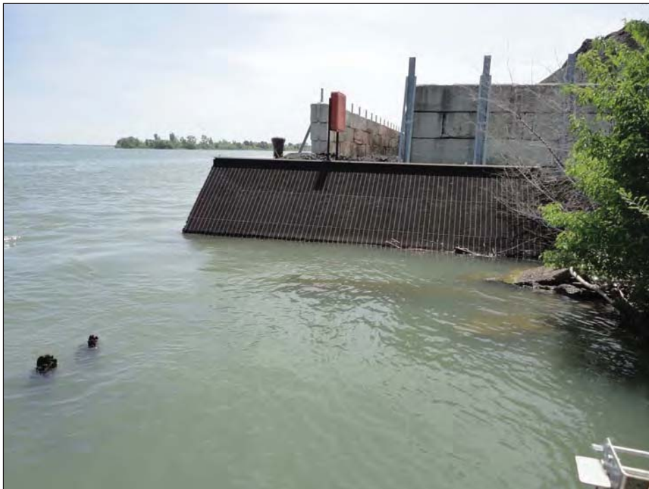
Wood pilings in broken concrete rip rap inlet
