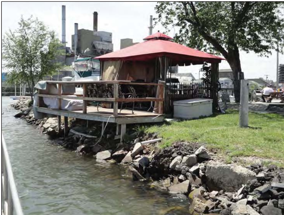
Broken Concrete Rip Rap with wooden deck/cabana structure
