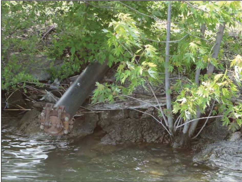
Broken Concrete Rip Rap and outfall pipe with cap
