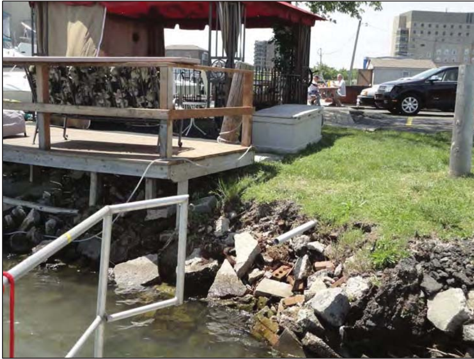
Broken Concrete Rip Rap with 2" outfall pipe about 3 ft north of wooden deck
