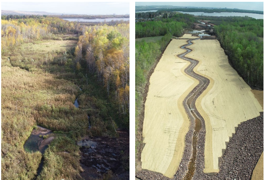
Site restoration highlight: Before (left) and after (right) remediation and restoration of the Unnamed Creek. Plantings along the channel and in the floodplain will be completed in early summer 2021.
