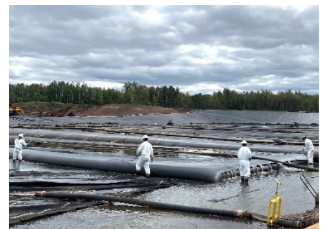
Dredge material from the Wire Mill Delta is pumped into Geotubes® in the Upland CDF.
