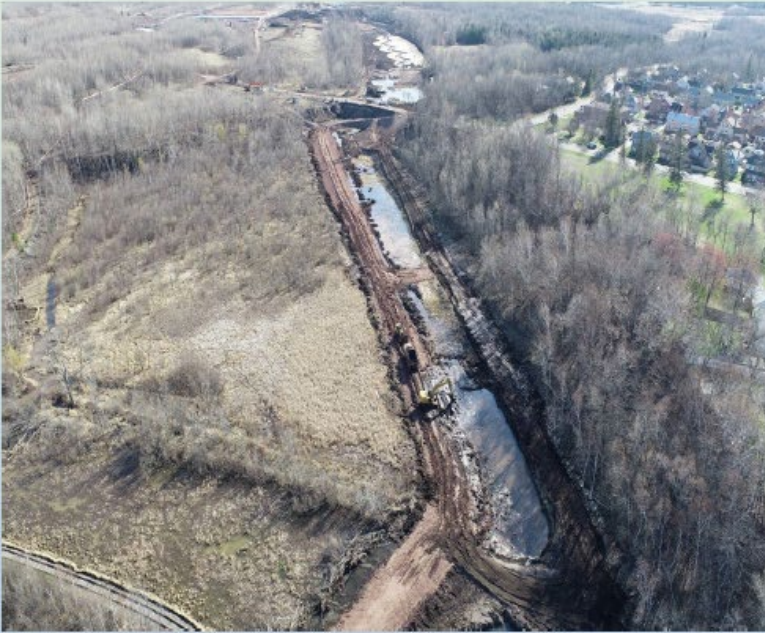
Before: Photograph of Upland CDF facing toward Spirit Lake in early construction stages.
