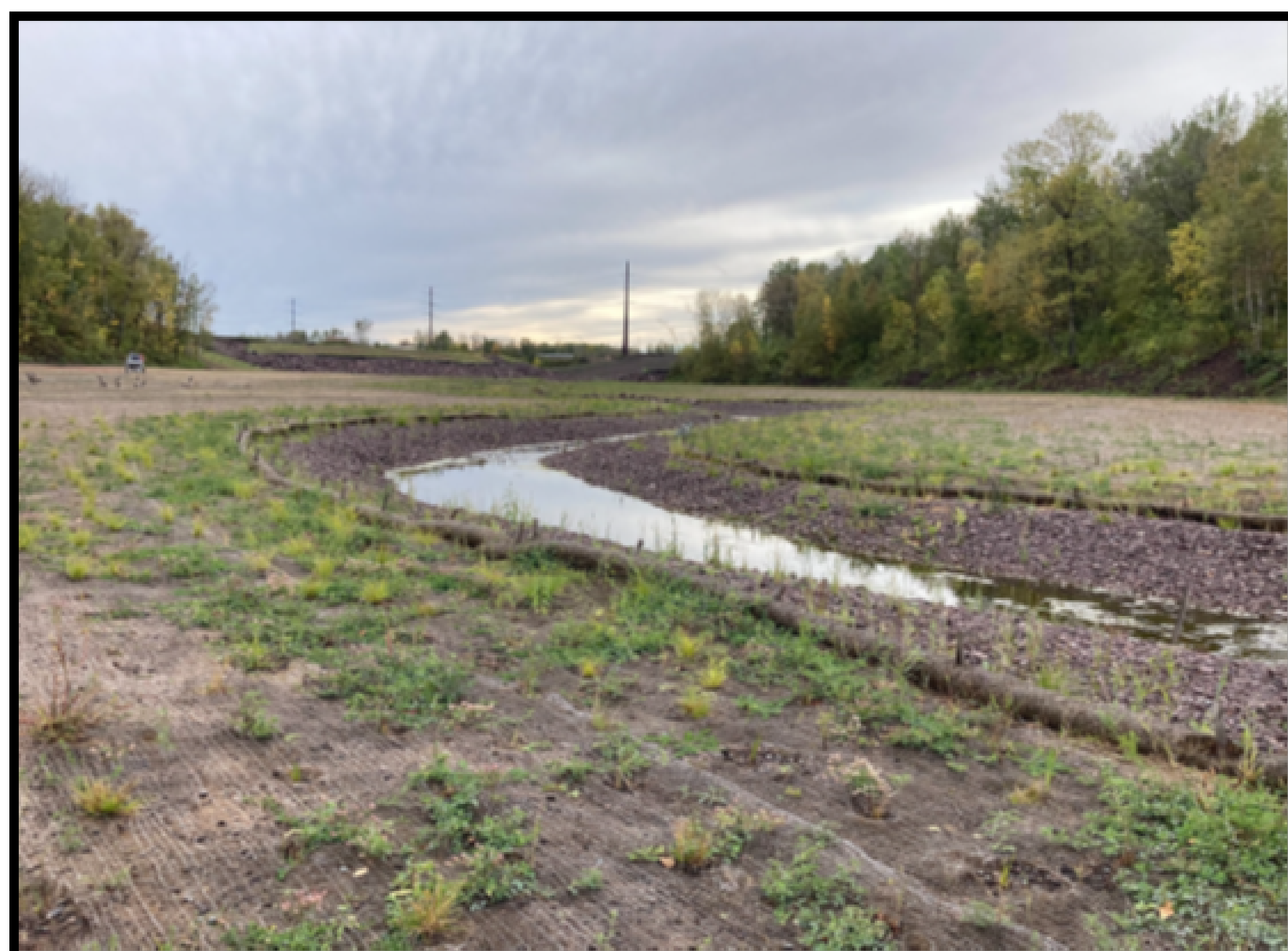
Unnamed Creek has been planted with riparian and emergent wetland species following remediation and rerouting in Summer and Fall 2021.
