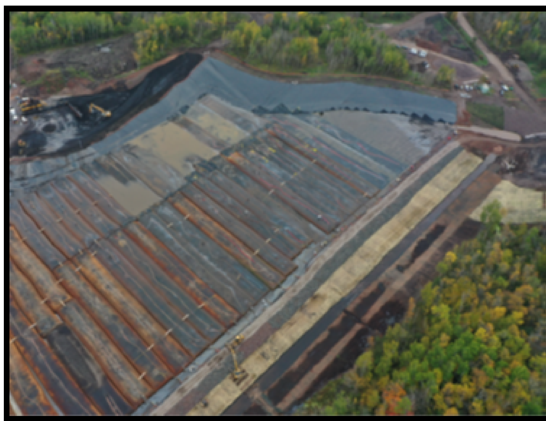
Dredge material is pumped into Geotubes® located in the Upland CDF. Geotubes® are specially engineered tubular, bag-like filters used to remove water from the dredge material before processing.
