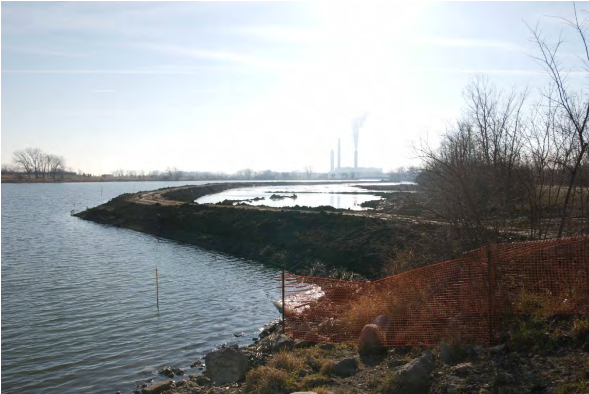
Looking South at the Temporary Dike/Haul Road at the Shallow Water Restoration at Sterling State Park
