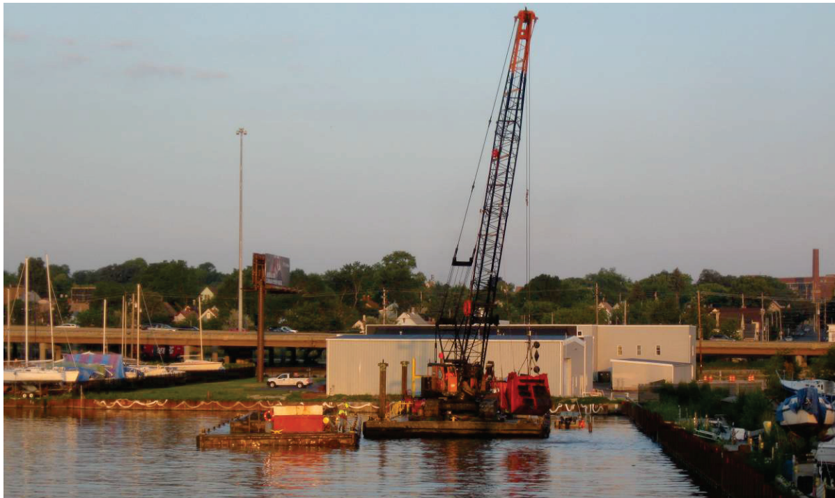
8. This photo shows Ryba dredging in the northwest corner of the project area.
