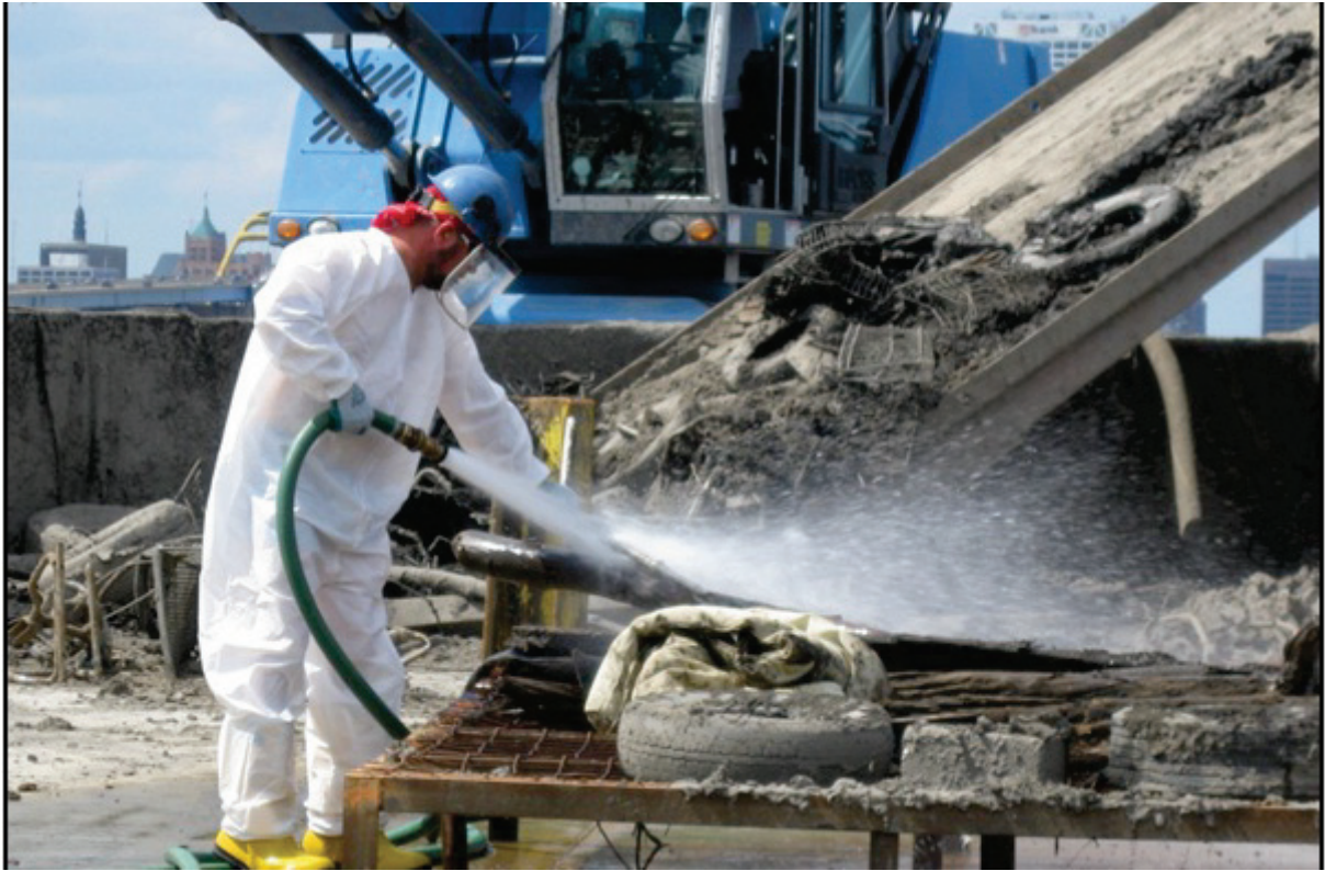
13. At the CDF, debris was screened, rinsed, and loaded into a rolloff box for disposal.
