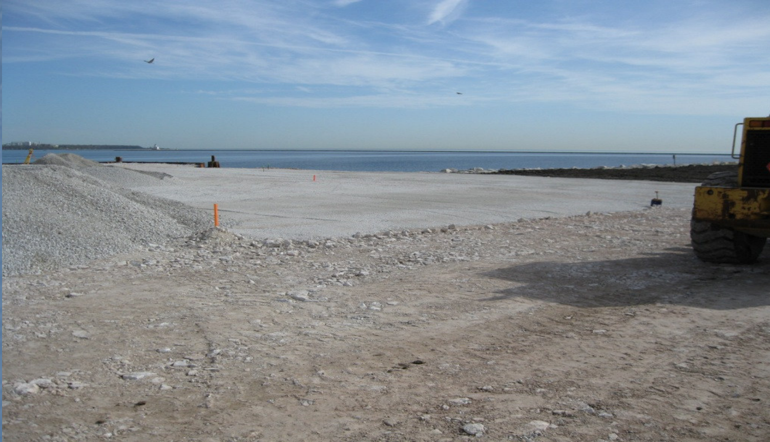
Offloading platform with sluice way sub-base compacted and at final grade (looking to the northeast).
