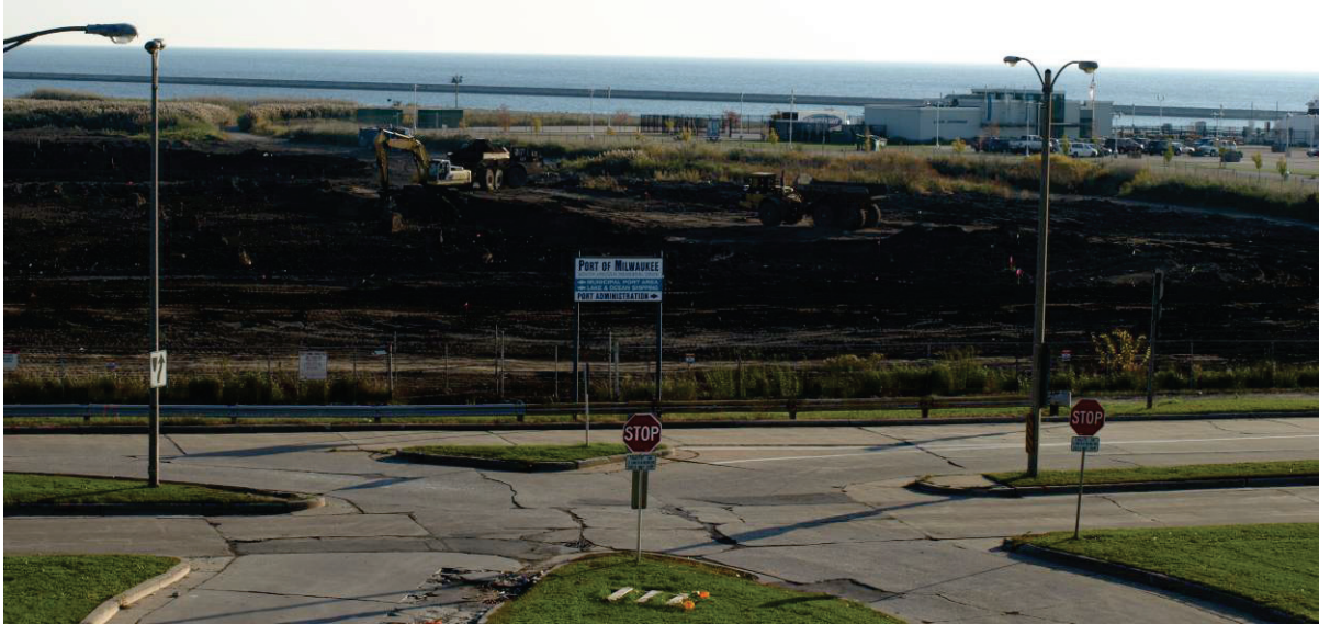
1. Freeman Environmental Services, Inc. (Freeman) and its lower-tiered subcontractor New Berlin Grading (New Berlin) constructed the cell at the CDF that contains the dredged material from the Kinnickinnic River.
