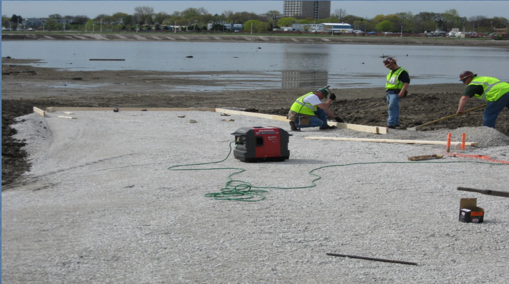
Forming for the construction of the concrete sluiceway (looking south from the offloading platform).
