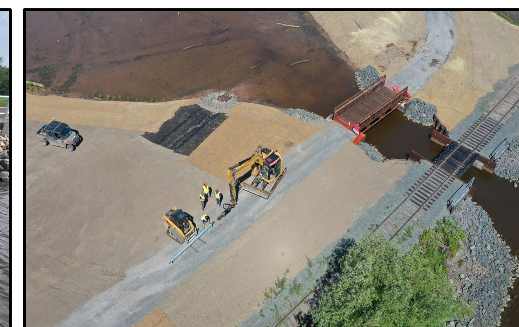
Posts to support the interpretive signage along the pedestrian trail are installed.
