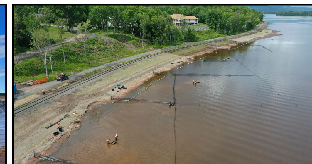
Planting is performed by hand installation methods along the shoreline of the SSB.
