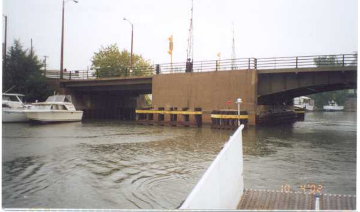
PHOTO 44 – October 4, 2002 – Kinnickinnic River Taken by Tor Hansen, Barr Engineering Upstream face of left abutment and pier of 1 st Street Bridge. Looking downstream or east.
