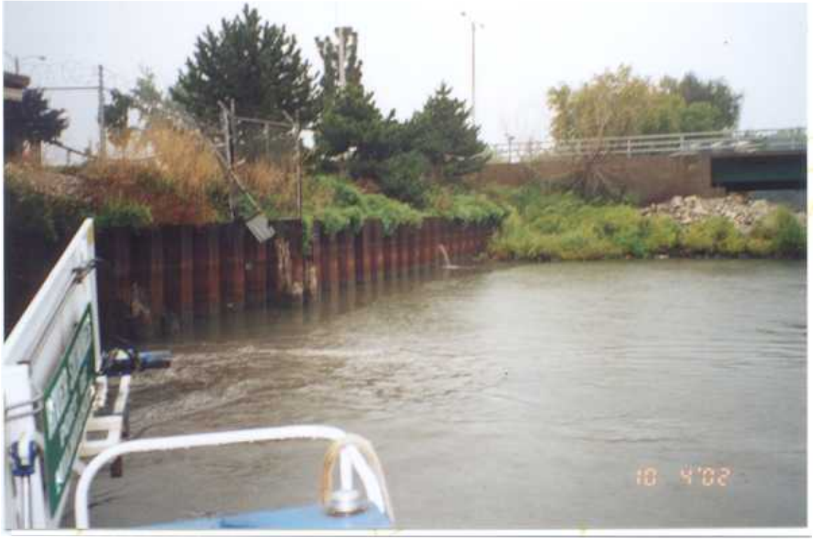
PHOTO 47 – October 4, 2002 – Kinnickinnic River Taken by Tor Hansen, Barr Engineering Steel sheet pile wall along Parcel 432 and upstream end of Steel sheet pile wall along Parcel 433. Looking southeast.
