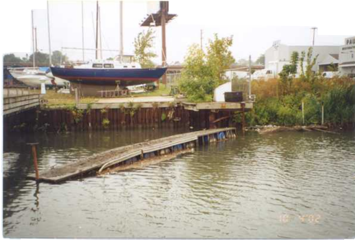
PHOTO 10 – October 4, 2002 – Kinnickinnic River Taken by Tor Hansen, Barr Engineering Downstream end of steel sheet pile wall along Parcel 429 and upstream end of Parcel 428 showing vegetative cover at shoreline. Looking west.
