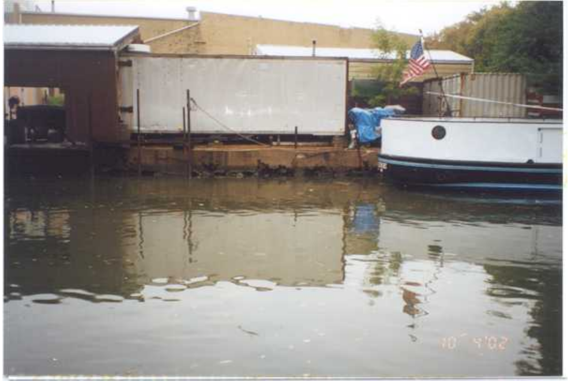
PHOTO 36 – October 4, 2002 – Kinnickinnic River Taken by Tor Hansen, Barr Engineering Concrete and timber wall along Parcel 425. Looking north.
