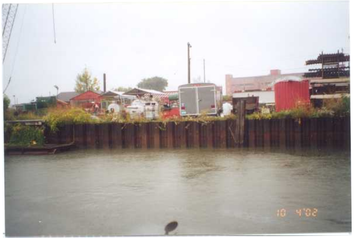
PHOTO 52 – October 4, 2002 – Kinnickinnic River Taken by Tor Hansen, Barr Engineering Steel sheet pile wall along Parcel 433. Looking east.
