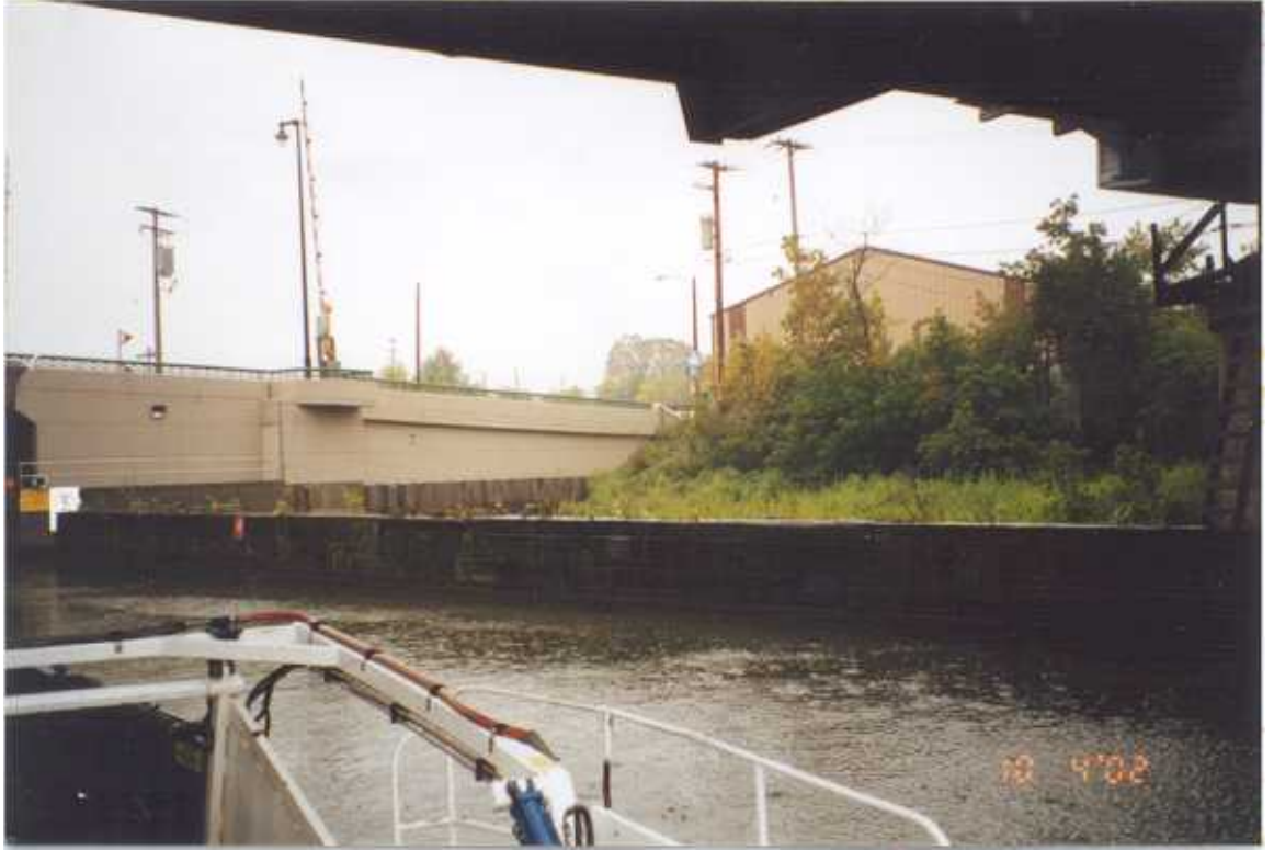
PHOTO 72 – October 4, 2002 – Kinnickinnic River Taken by Tor Hansen, Barr Engineering Timber pile fence protecting bridge pier adjacent to Parcel 443. Looking south.
