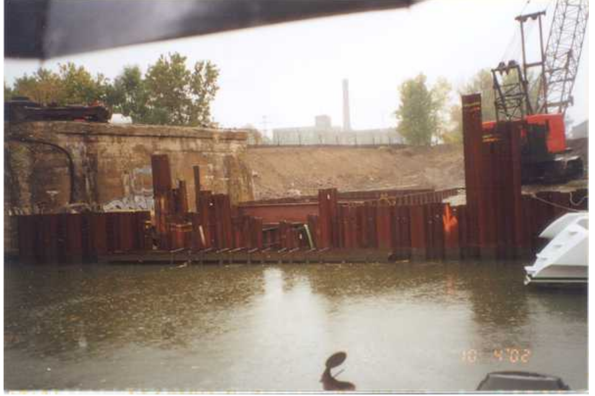
PHOTO 68 – October 4, 2002 – Kinnickinnic River Taken by Tor Hansen, Barr Engineering New steel sheet pile construction adjacent to old bridge abutment at Parcel 440. Looking south.
