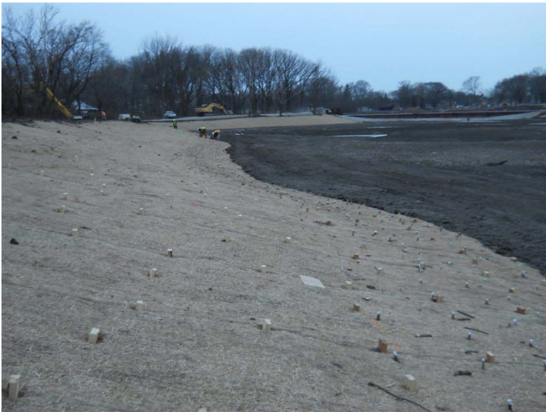
Figure 14: Coir blankets placed/staked and live stakes planted north bank of Zone 2A (12/8/2011)
