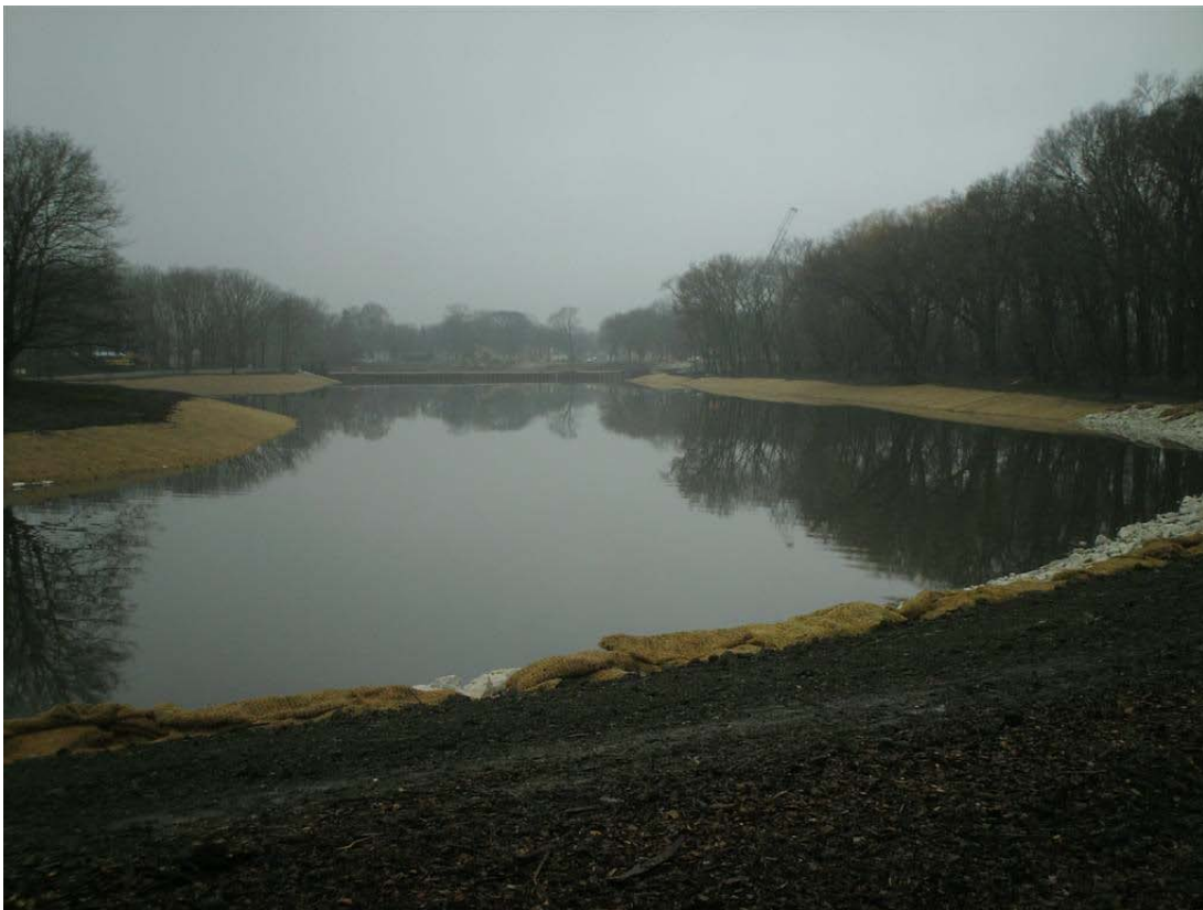
Figure 15: Water flow from Lincoln Creek was redirected through Zone 2A from Zone 2B (12/14/2011)
