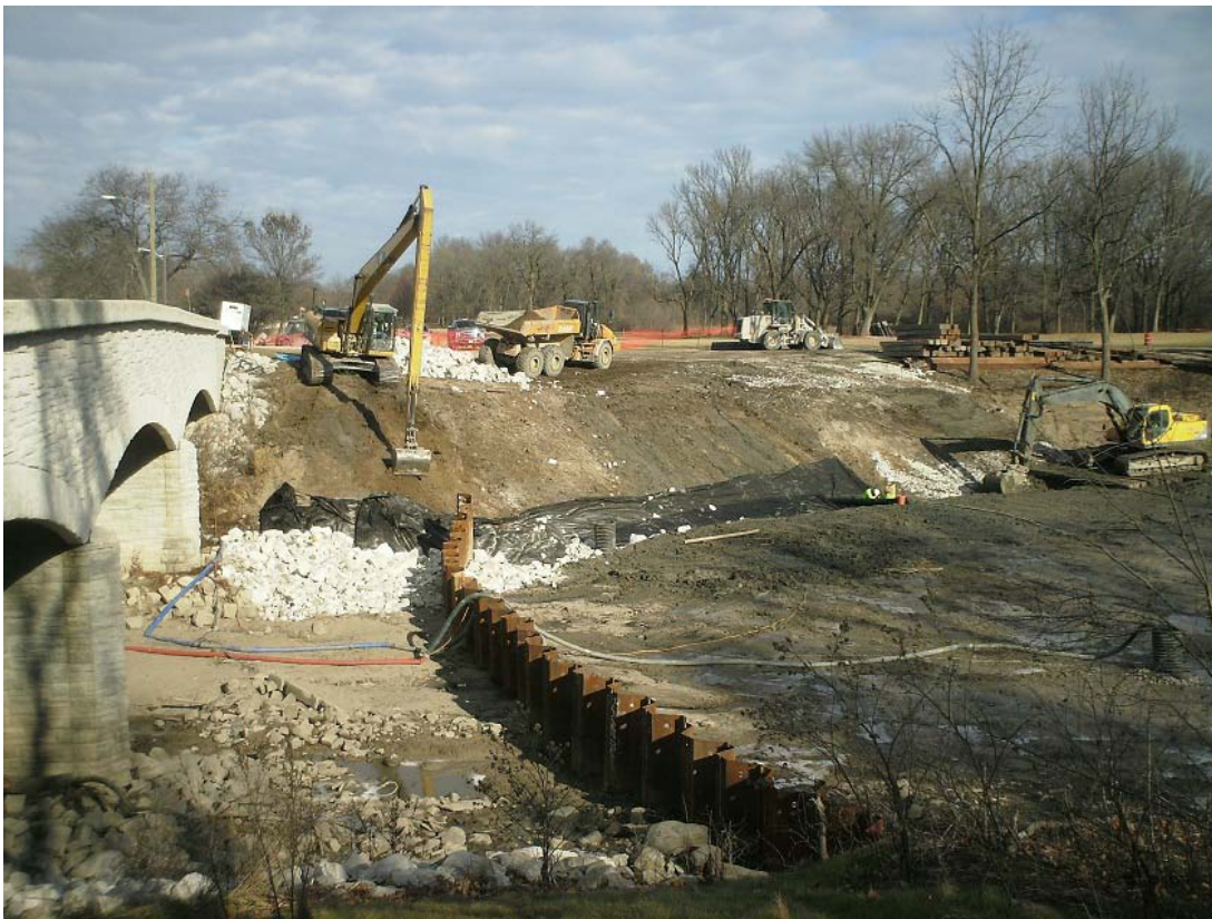
Figure 18: Restoration begins on the north bank on Zone 3A, trenching keyways, placing fabric and riprap (1/9/2012)
