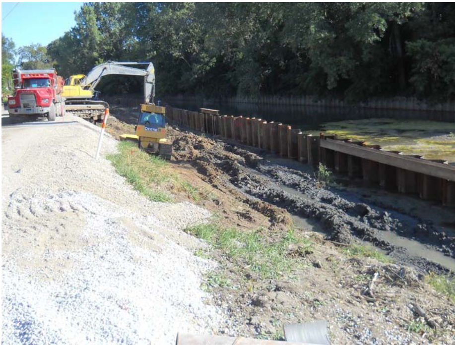
Figure 5: Excavation work in the west side of Zone 1 north of the tower access bridge (9/15/2011)
