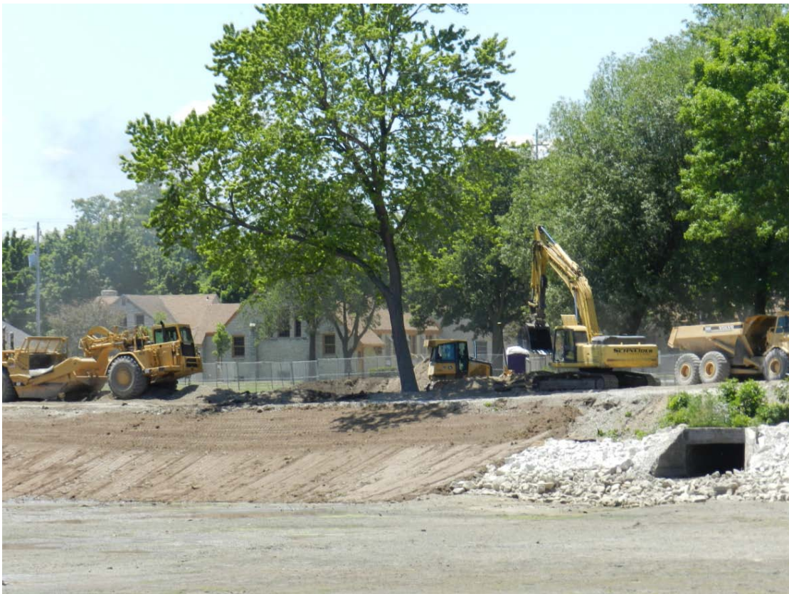
Figure 20: Restoration of west slope of Zone 2b; Removal of temporary road and decontamination pad on the west slope of Zone 2b
