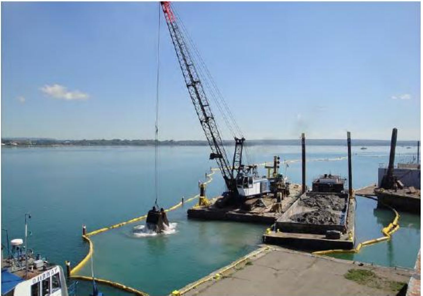
Dredging with machinery like this cable arm environmental clamshell bucket moved 24,000 cubic yards of contaminated sediment out of the St. Marys River.
